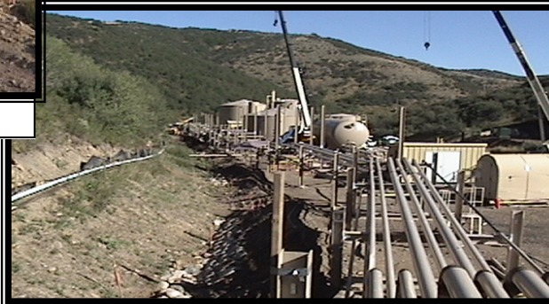
Piping system, Wilson Creek, Colorado.
